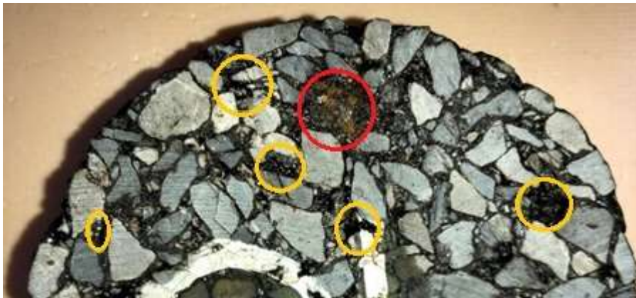
Figure 10 PFC specimen #16 showing localised issues of oxidation and binder damage.
